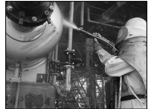
Knight Industrial's mobile, multicraft crews have helped pipeline companies such as BP, ExxonMobil and Enterprise Products get more bang for their buck.
